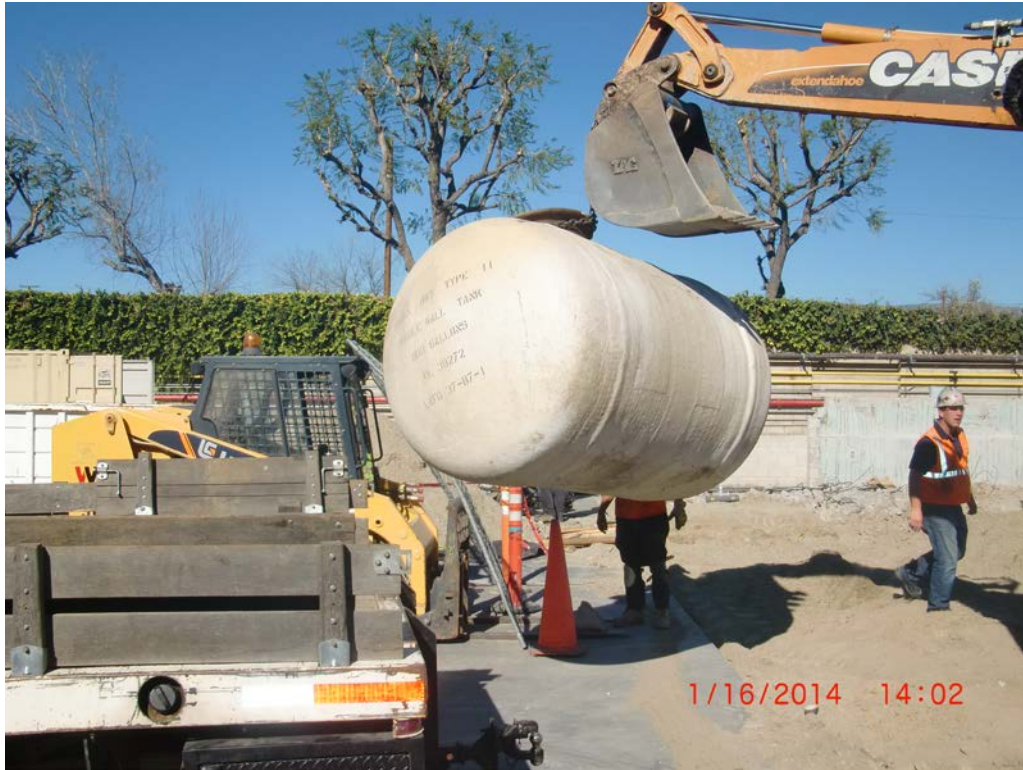
1. Removal of the 600 Gallon Underground Diesel Tank (Last of Underground Tanks removed from VMF Property – 8 Tanks Total).
