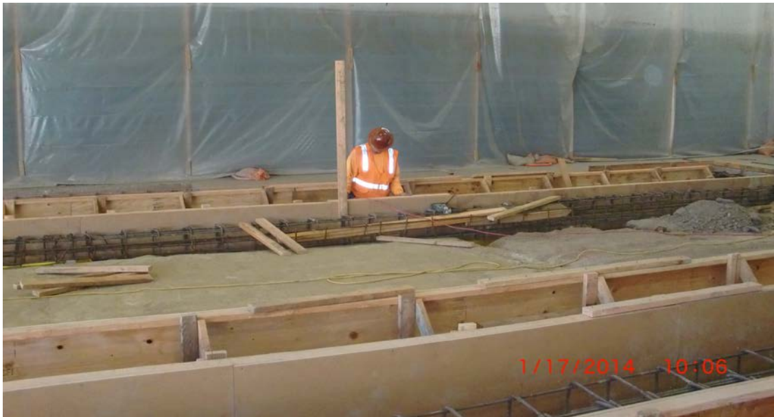
2. Placing Rebar and Installing Formwork for Bus Lift Pits in Maintenance Facility (Building A).
