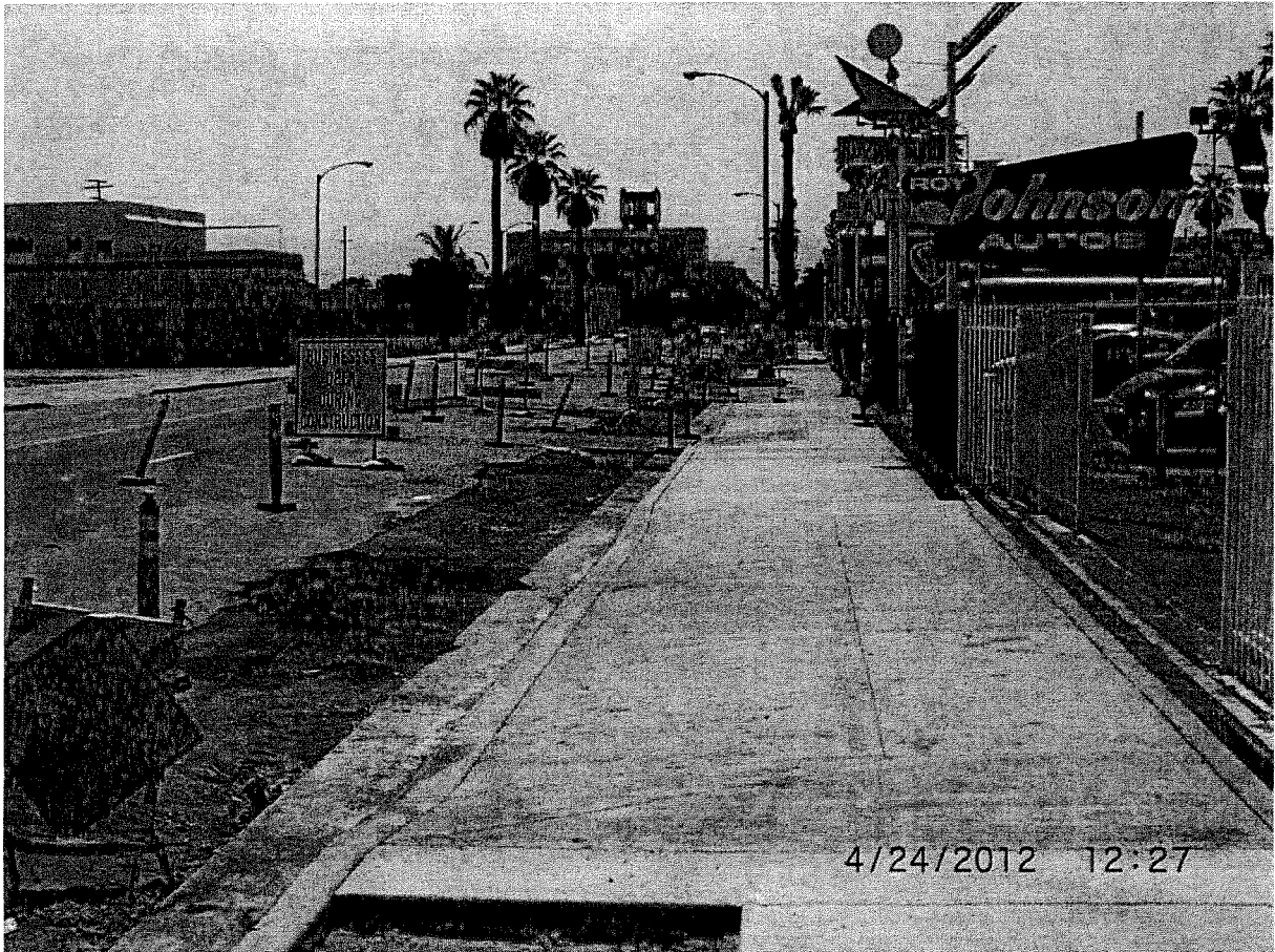
New curb, gutter, driveways & sidewalk along E Street, looking south between 9 th and Union Streets
