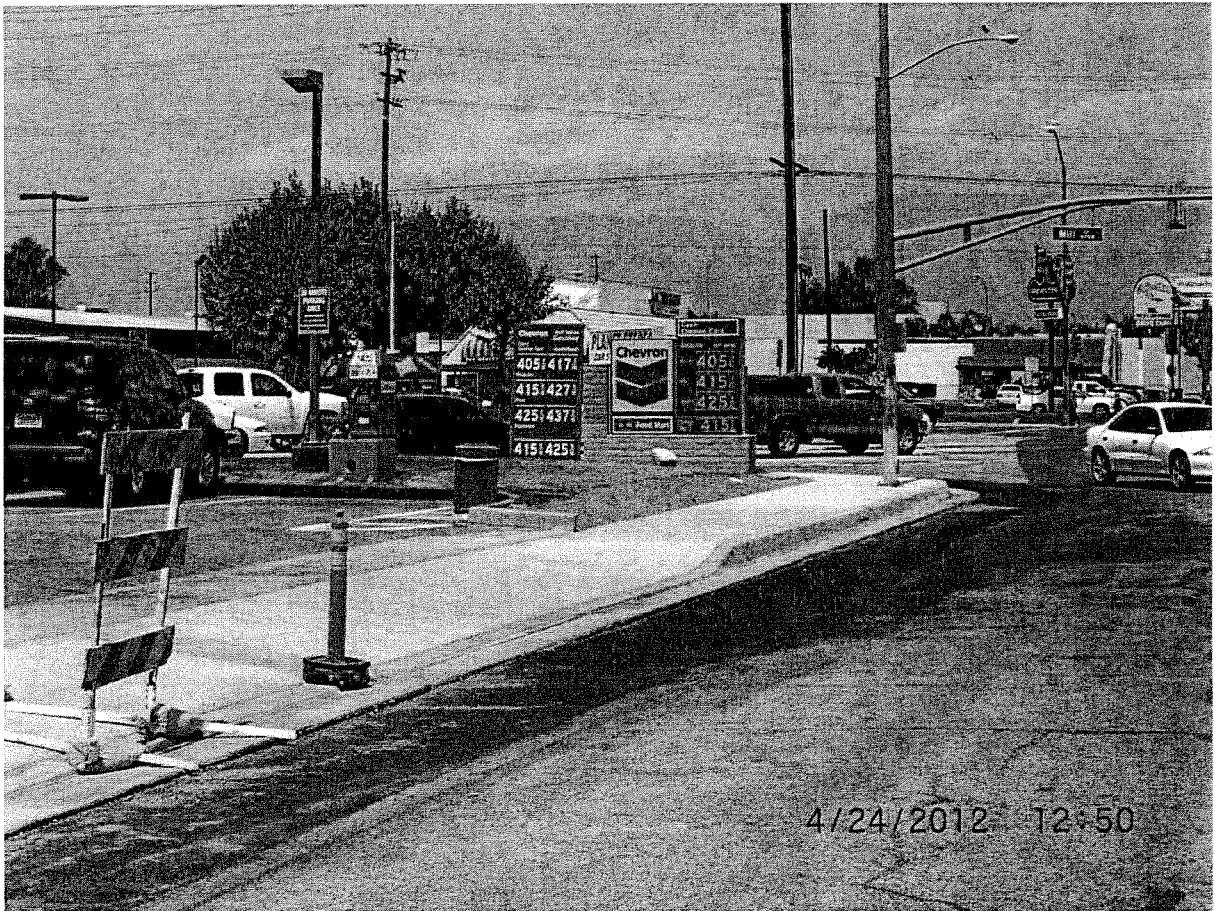
New curb, gutter, driveway & sidewalk and relocated signal pole at SW corner of E Street & Inland Center Drive looking north
