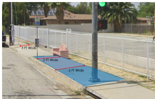
The landing pad does not adhere to ADA standards. Additionally, the bench partly obstructs it. The path of travel is narrow and cramped, and the sidewalk is not very accommodating.
