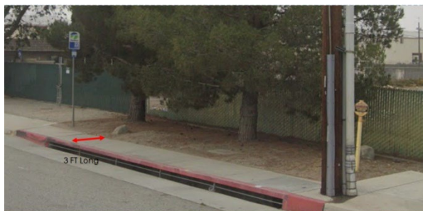
Landing pad is less than 3 ft wide.
